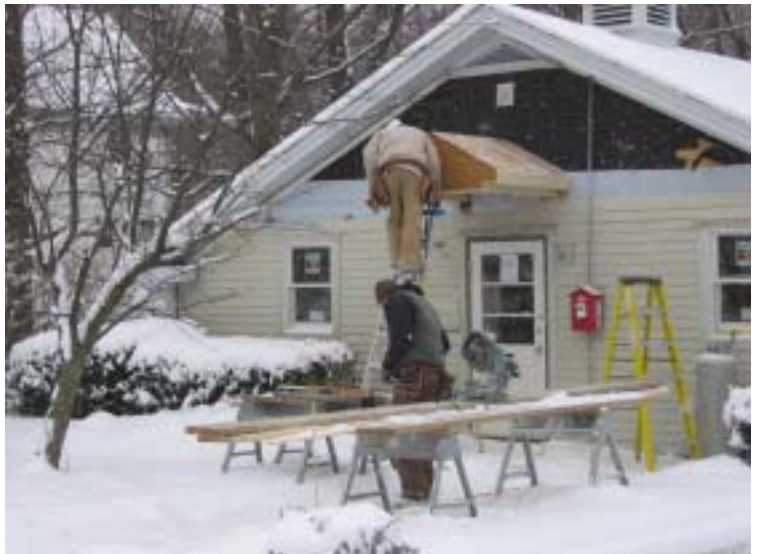
Light snow didn't stop workers from American Construction renovating the upstairs of 44 Concord Street.
